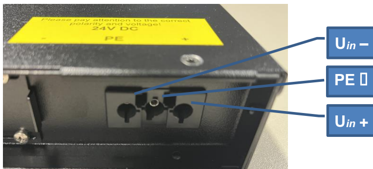
Figure 11: DC voltage connection at the power supply
